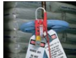
Lockout gate valves
