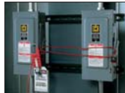
Lockout single or multiple electrical disconnects
